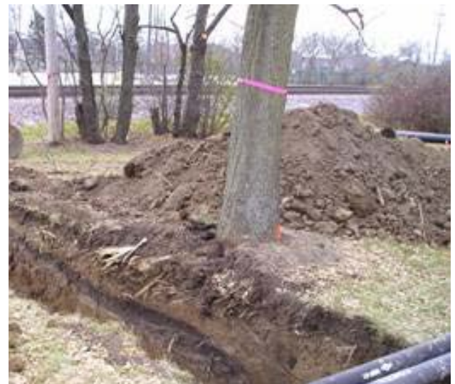
Fatal root damage due to trenching within root zone
